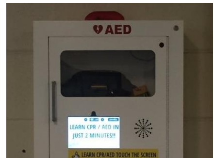
“Smart” AED Cabinet
